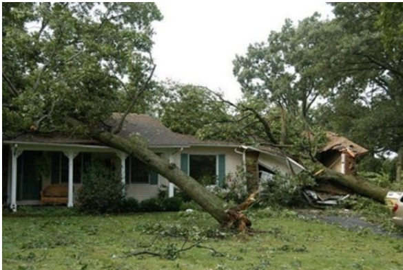
Figure 22 Home Damaged During Windstorm
