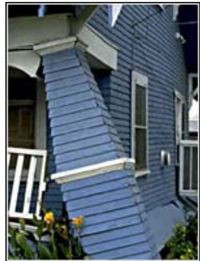
Figure 10 Earthquake Damaged Porch
