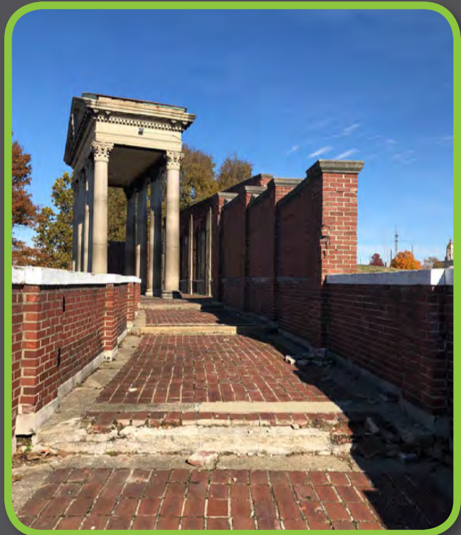
Memorial at Fairbanks Park in Need of Repair
