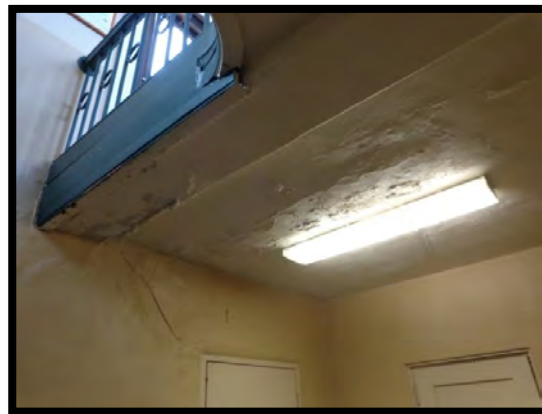
Cracking in Basement Walls & Ceilings
