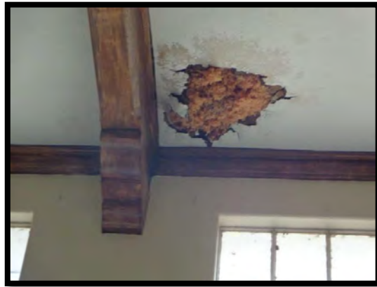
Water Damages in Main Hall Ceiling
