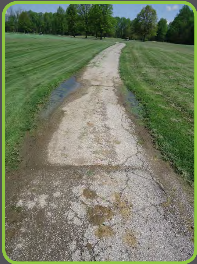
Cart Path in Poor Condition
