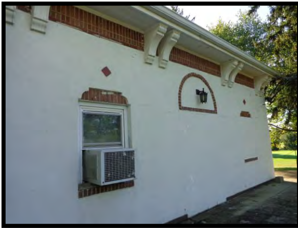
Windows Blocked Shut
