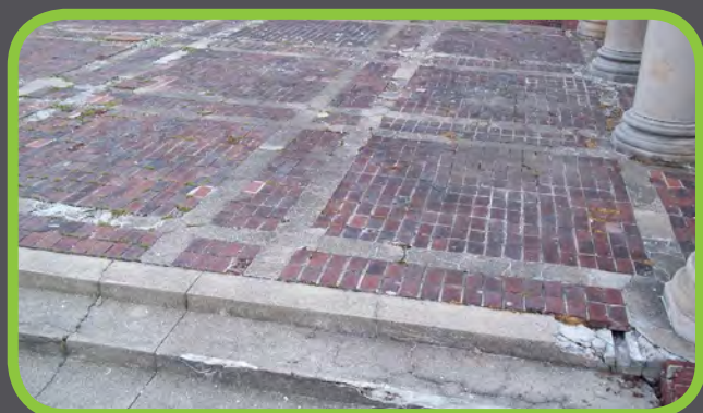
Brick work in need of repair
