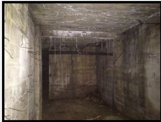
Water Damage Under Westside Terrace
