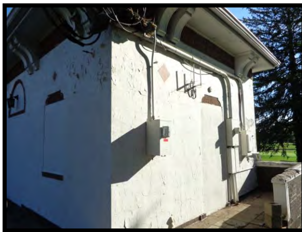
Outside Electrical Boxes
