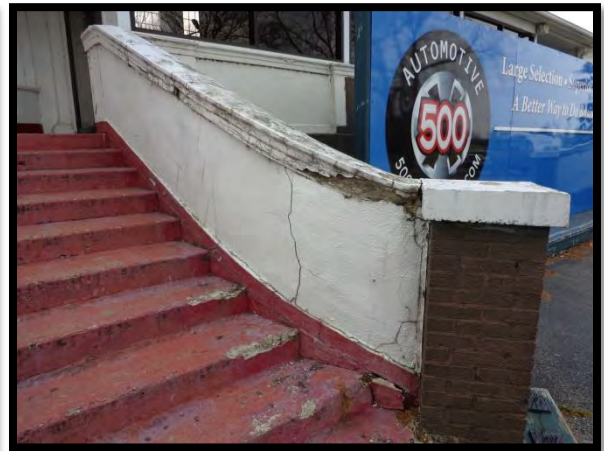
Deteriorating Steps on the East Side
