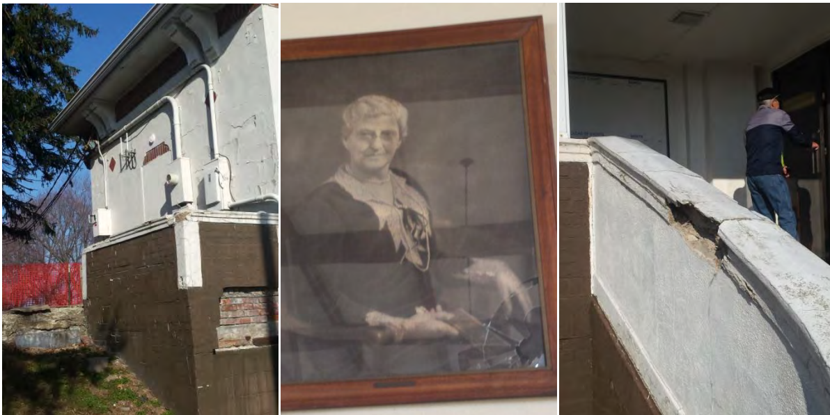
L to R: South side of clubhouse, Mrs. Rea's damaged portrait, crumbling east side stairway
