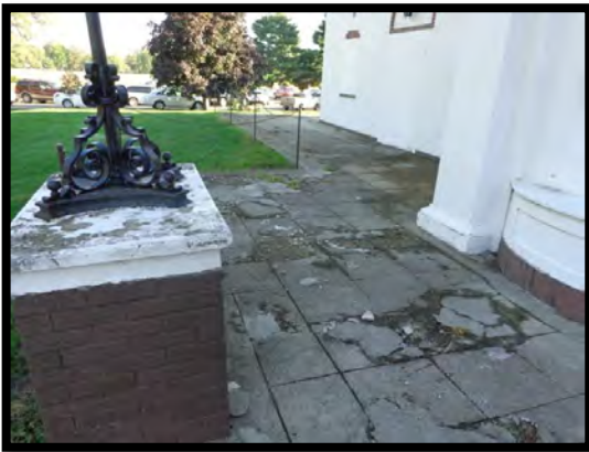
Deteriorating Westside Terrace
